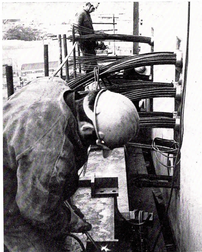
Work prior to final tensioning of cables in Western Concrete Approach Viaduct.
