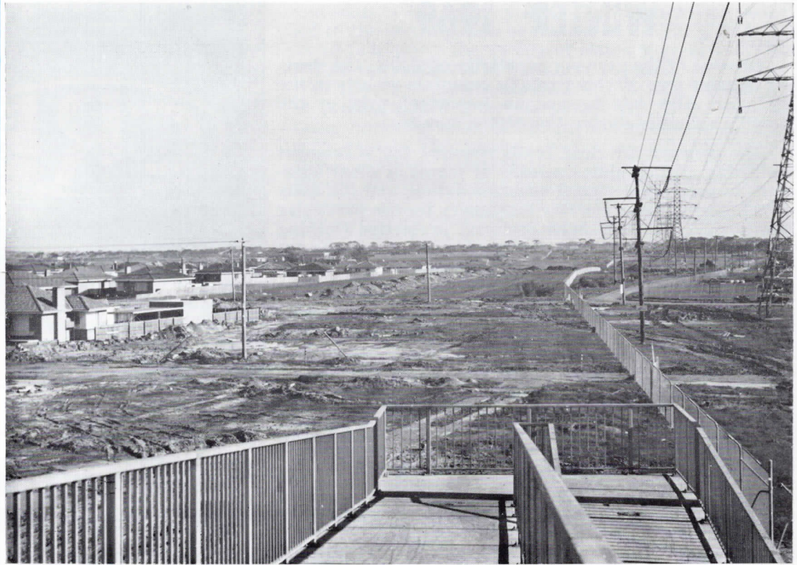
View of Lower Yarra Freeway route looking west from Rosala Avenue, Brooklyn with pedestrian overpass ramps in foreground.
