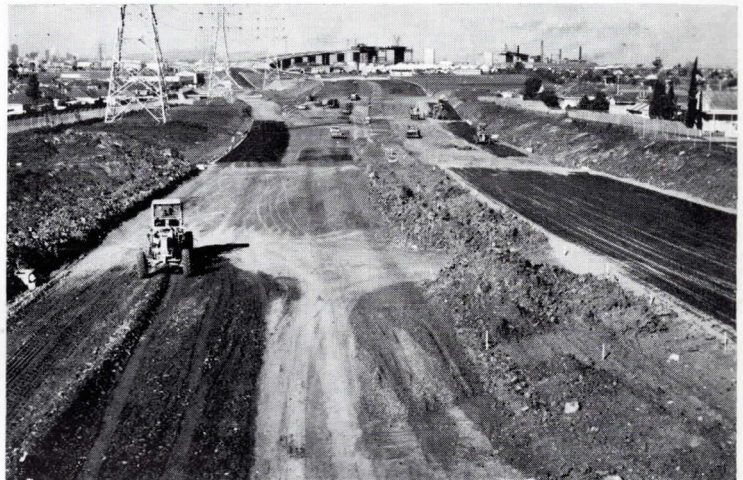
Progress on the Lower Yarra Freeway. Looking east towards the Williamstown Road interchange.
