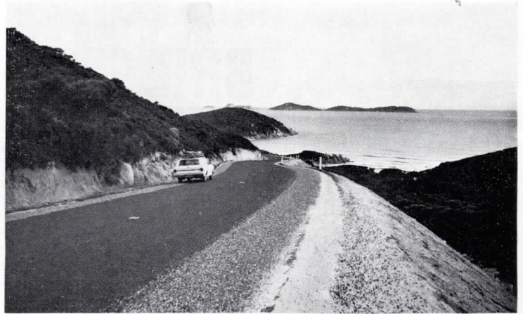
Wilson's Promontory road has recently been improved by the C.R.B. It now plans a continuation of the reconstruction of over 3 miles between Darby River and Tidal River.
