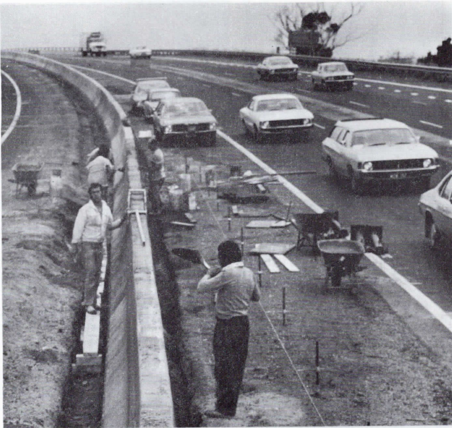
Section of the new median barrier safety wall being constructed along 8 kilometres of the Princes Highway (Geelong Road) at Laverton, Victoria.
