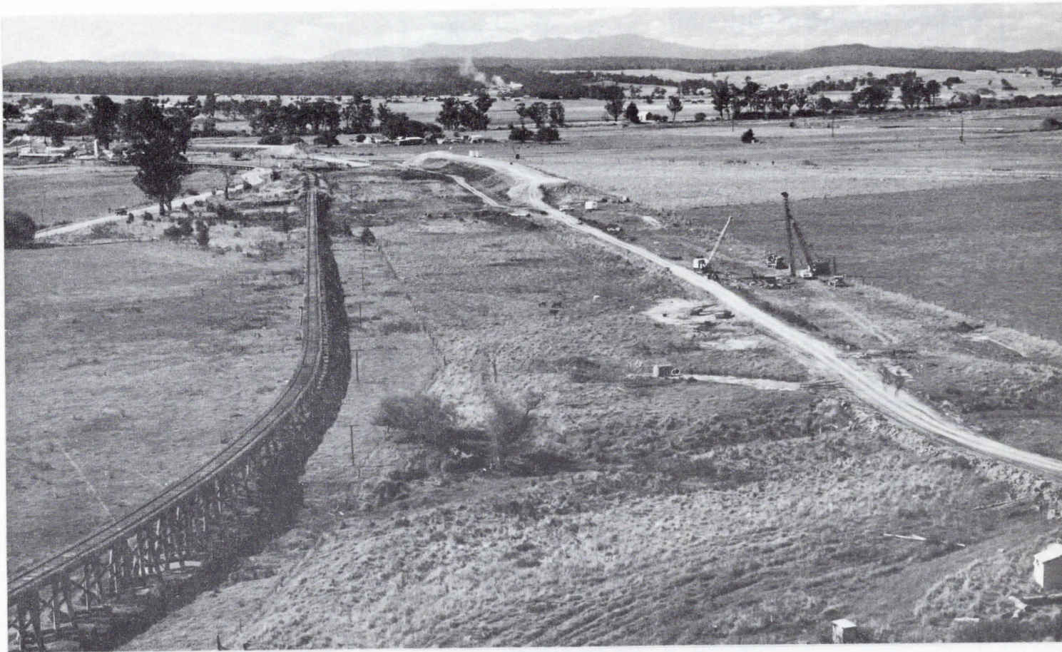
The Snowy River flood plain at Orbost, showing the railway bridge (left), and the general alignment of the new road bridges under construction.
