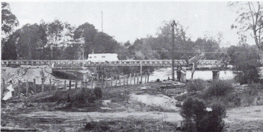
The old road bridge over the Cann River at Cann River is being removed to make way for a new bridge. A temporary bailey bridge has been erected to carry traffic using the Princes Highway East.
