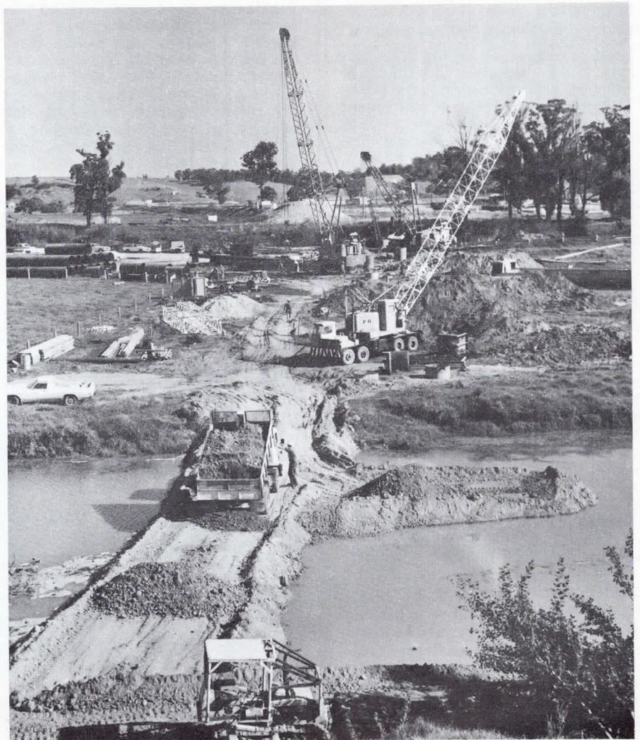
Pile driving in progress on the east bank of the Snowy River at Orbost. The water in the foreground is a billabong, which, with the main river channel, will be spanned by a bridge 366 metres long.
