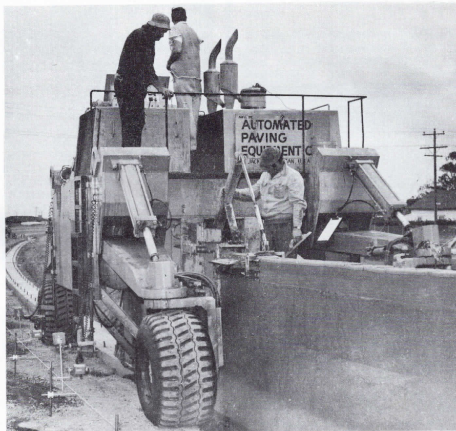
A $100,000 automated concrete slip-forming machine was used to build a new median barrier safety wall along 8 kilometres of the Princes Highway (Geelong Road) near Laverton.
