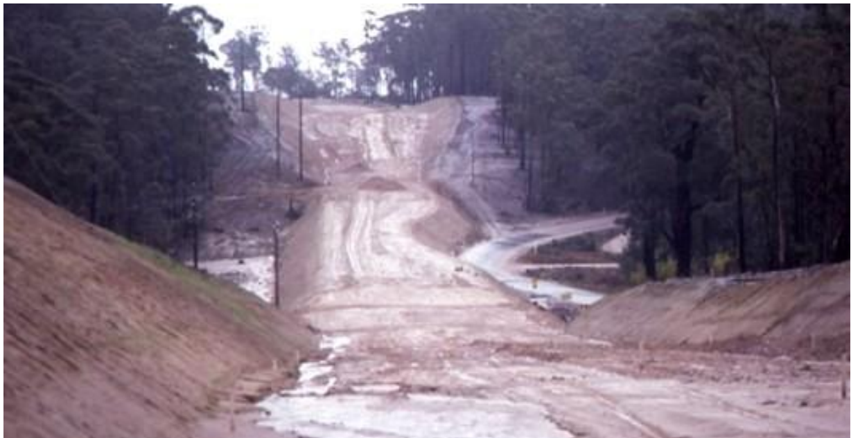
Rain Damage on the Simpsons Creek project
