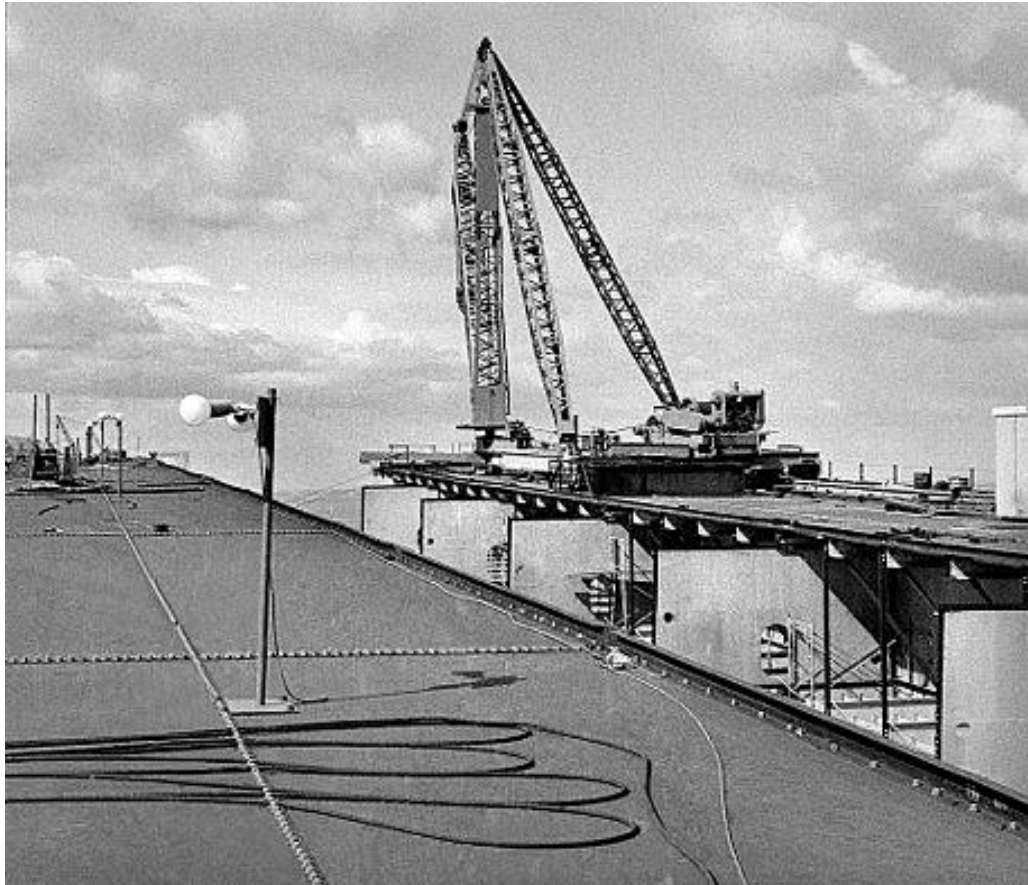
Looking east on Span 10-11. The crane is on the southern half, which has just been jacked up from ground level and it will be rolled towards the northern half where the photographer is standing. The undulating upper edges of both halves are evident. The stiffening of the deck plates is also evident. (Image courtesy of Rob Morgan ARPS)
