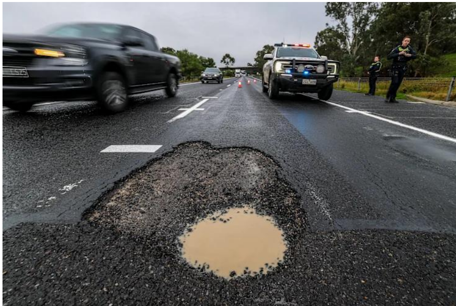
A pothole on the Hume Highway recently caused five cars to suffer flat tyres in rapid succession.
